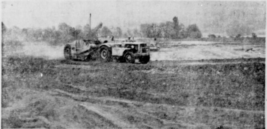
The Kuckenber Construction company has nearly brought to completion a mill pond covering some 15 acres of land area. The pond shown in the construction stage above is located near the Apple Tree Court on the North Santiam highway near the railroad right-of-way. The pond will be used in connection with the plywood plant being constructed on the site by Idanha Veneer. Vern Alvin, manager of Idanha Veneer, states the plywood plant will be completed by April 1952. The new plant reportedly will employ some 60 men when operating. A fleet of "cats" and assorted earth-movers threw up the earth walls of the 15-acre pond. Shown above is a two-piece earth-mover releasing a load of scooped up soil atop the rim of the nearly complete pond. Water from the North Santiam river will be used in filling the pond. (Photo courtesy of The Statesman and Robert Venes)
