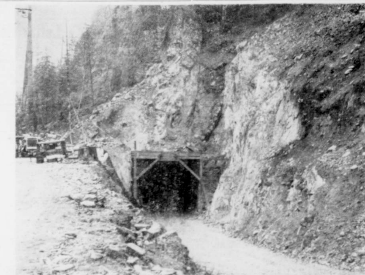
Big Cliff Dam diversion tunnel is nearing completion. Shay Construction company is pushing through the construction of this tunnel. Big Cliff diversion tunnel will carry the flow of the North Santiam River while construction work on Big Cliff Dam proceeds. The 600-foot long tunnel is 28 feet in diameter. It probably will be complete, July 18. June 29 is the deadline for submission of bids for the construction work of Big Cliff Dam, the regulating and power dam located three miles below Detroit Dam.
