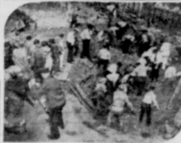
CAVE-IN FATAL —Rescue workers dig in search of workmen buried under tons of debris in a cave-in, at an excavation in Atlanta, Ga. Seven victims were dug out alive and four were dead.
