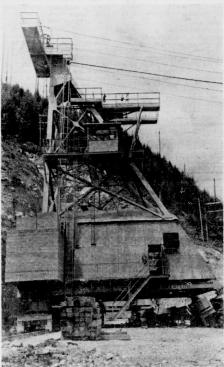
View of the cable way tower in use at the Detroit dam project on the south wall of the canyon. This cable way is capable of lifting a load of 25 tons of concrete and placing it anywhere within the dam base. It is the bearings used in this tower becoming "hot" that has been causing some trouble until they become broke in. A number have had to be replaced. However, the operation has been meeting all expectations and pouring of concrete is ahead of the mapped out schedule at this date, according to Russell Hoffman, CBI engineer in charge of operations. (Photo Courtesy Capital Journal)
