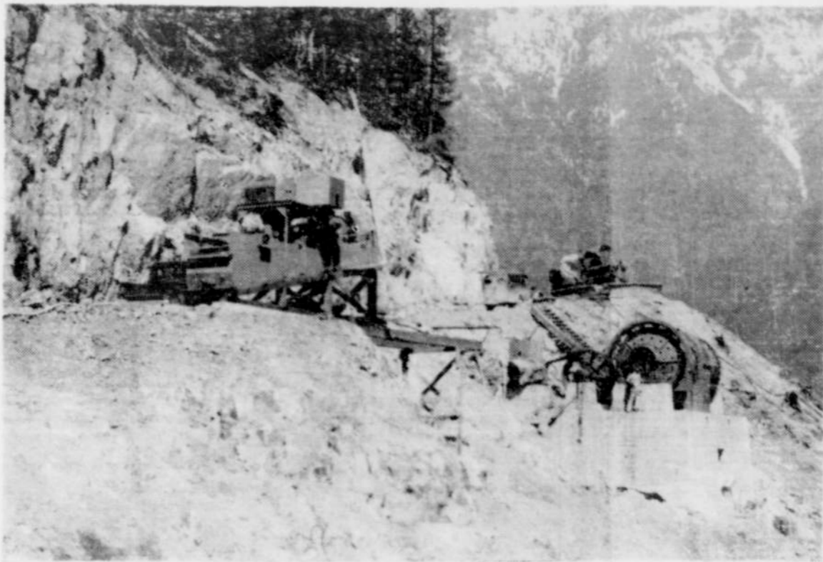
ROD MILL AND CLASSIFIER FOR DETROIT DAM—Machinery now being installed just above the aggregate storage plant at Detroit dam will function as a rod mill crushing rock into sand and operate as a classifier sorting rock of various sizes. Photo Courtesy Capital Journal.
