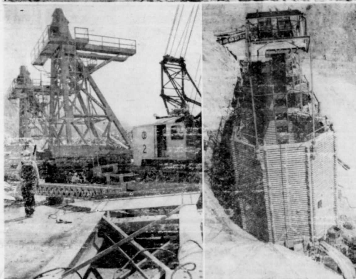
DETROIT DAM NOW 15% COMPLETE.—Top: Excavation for dam foundation and stilling basin where Consolidated Builders, Inc., have heavy machinery removing rock in the old Santiam channel. Lower, left: Towers on abutments above the dam will sustain cables carrying buckets of mixed concrete when pouring gets under way. Right: Storage plant for various sizes of aggregate and sand required for dam construction. Photos Courtesy of Capital Journal
