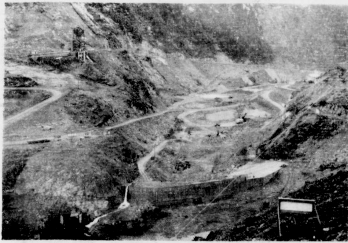
ALL IN READINESS FOR DETROIT DAM CONSTRUCTION—View looking down stream on virtually dry North Santiam river bed where Consolidated Builders, Inc., and army engineers are preparing to begin construction of huge Detroit dam. In lower left entrance to diversion tunnel through which the North Santiam is being diverted is shown. Immediately in foreground is coffer dam blocking progress of river. Spotted snow can be seen on side of hills.
