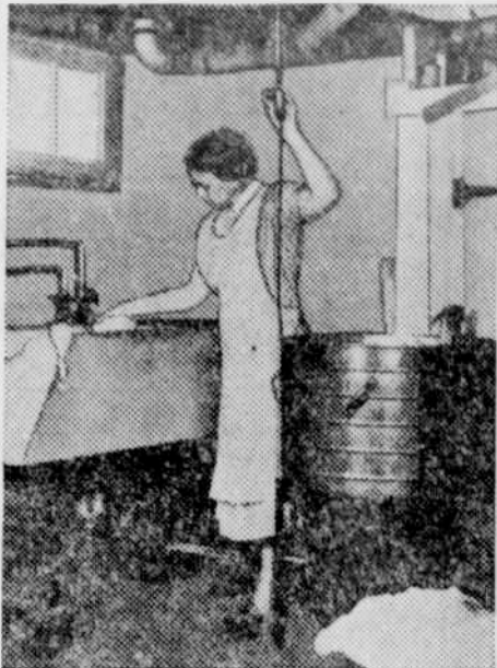
Washing machines must necessarily be used in the vicinity of water so that special precautions are advisable. Convenience outlets with insulating covers are preferred to pendent cords. Metal sockets as shown here should not be used in this location.
