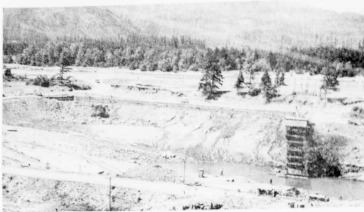
General view of the site in the south channel where power house excavation is rapidly nearing completion by the Guy F. Atkinson company. Bradford Island is shown in the background. In the foreground is shown the road over which President Roosevelt will drive today while inspecting dam.
