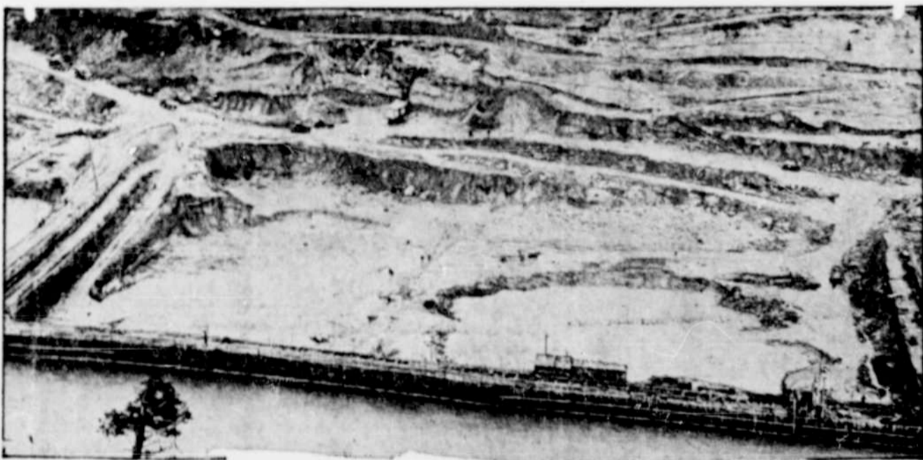
The excavation work for the first half of the dam base is well under way, as shown in this new picture of the Norris Dam project in Knoxville. The excavation work extends about fifteen feet below the river bed, and digging will be continued until solid rock is reached.
