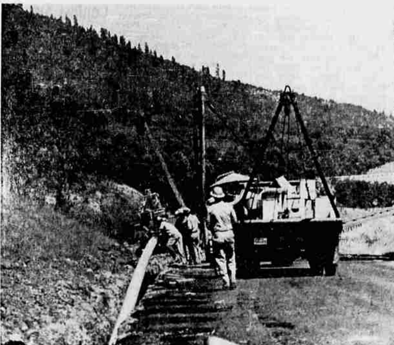
Pipeline installation was the first step in bringing natural gas to Southern Oregon.
