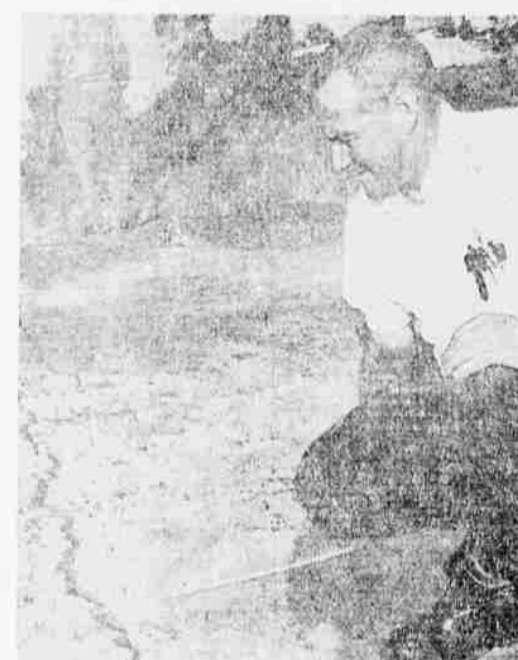
CRACK INSPECTED — Water Service Chief Lee Clark inspects a crack in the surface of the Baldwin Hills reservoir dam just prior to the disaster. This crack was the first warning officials had of what was to come. Rescue and cleanup crews were swarming over the area today in attempts to get accurate estimates of loss of property. (UPI)
