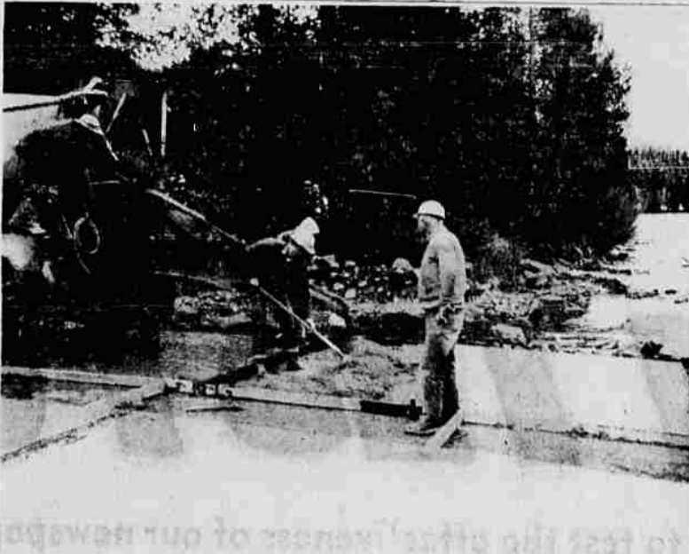
POUR CONCRETE — Forest Service crews are shown here pouring concrete for a new boat ramp at Diamond Lake. The work was financed through the Accelerated Public Works program.
