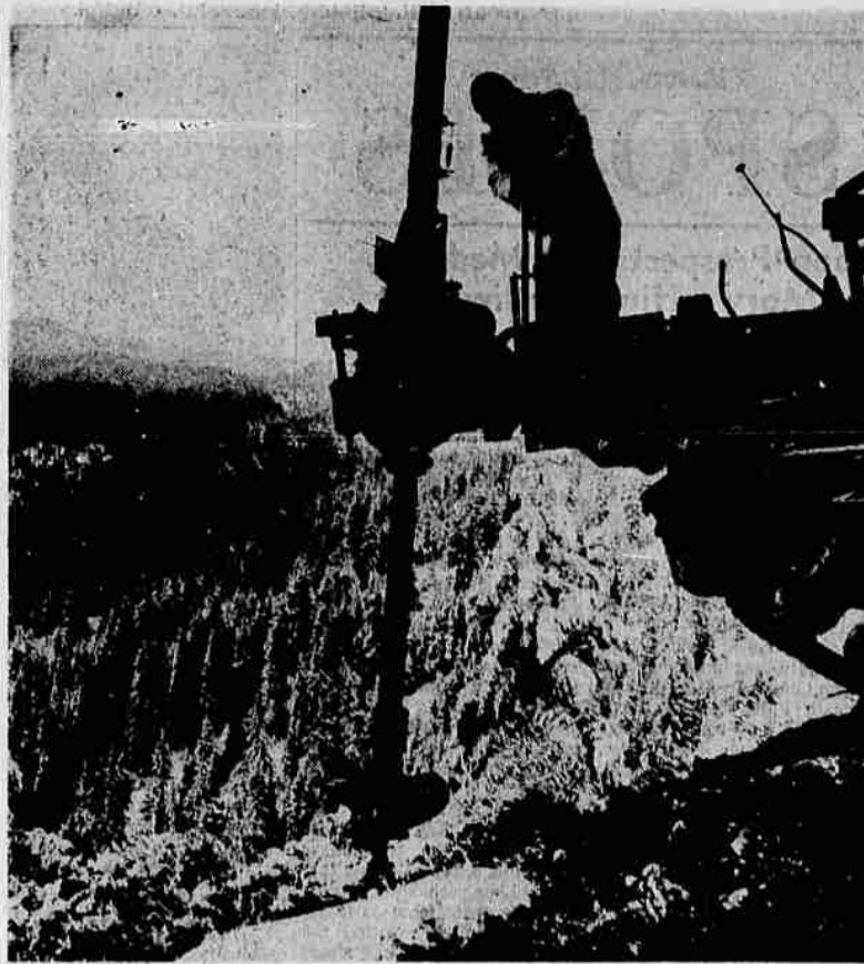
MT. ASHLAND PROJECT — A PP&L construction worker drills a hole for a power pole along the snow-cloaked route of Pacific Power's new 12,000-volt distribution line to serve the Mt. Ashland winter sports resort.
