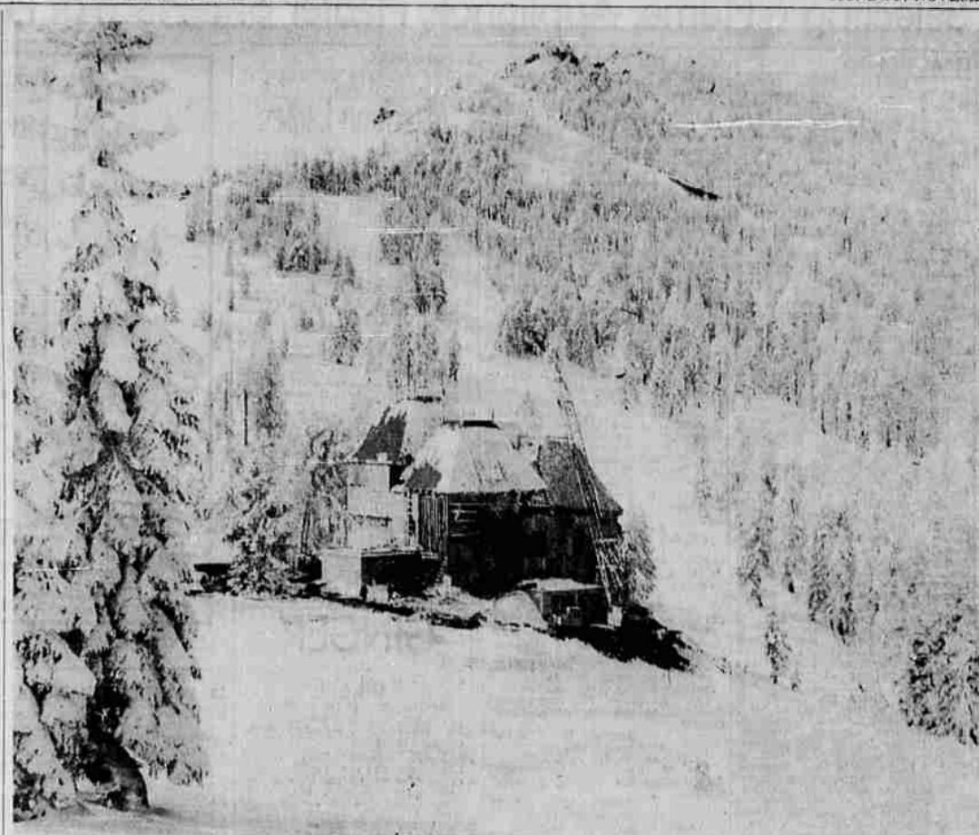
ALMOST READY FOR SKIERS—Two feet of snow now cover the slopes of the Mt. Ashland Ski Area as workmen rush to complete the lodge in time for this winter's ski season. In this photo, taken in the latter part of the week, the large crane brought in from Eugene may be seen as it placed the fourth of four towers into place atop the lodge. All that remains now to cover the top of the building is the installation of a chimney, expected to be done sometime this week. Ultimately, much of the lodge walls will be in plate glass, but for this winter a temporary wall of plywood and fibre-
