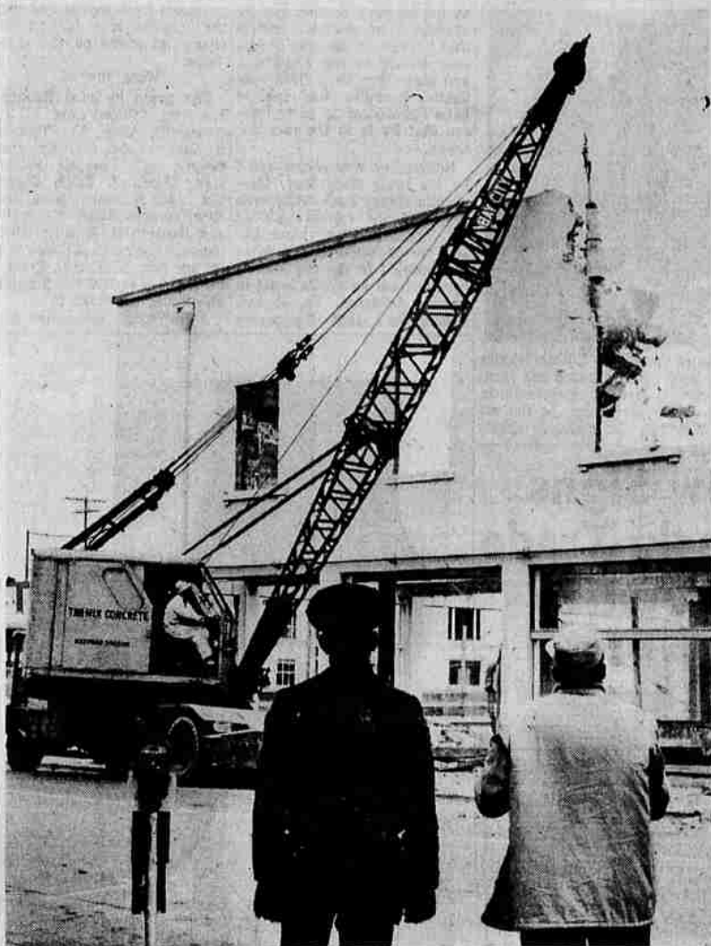
SMASHES WALL — As onlookers watch, demolition crews began razing the outer shell of the Hansen building at Sixth and Bartlett Streets Monday. Contract for the demolition work on the structure, as well as the old Federal building at Riverside Avenue and
