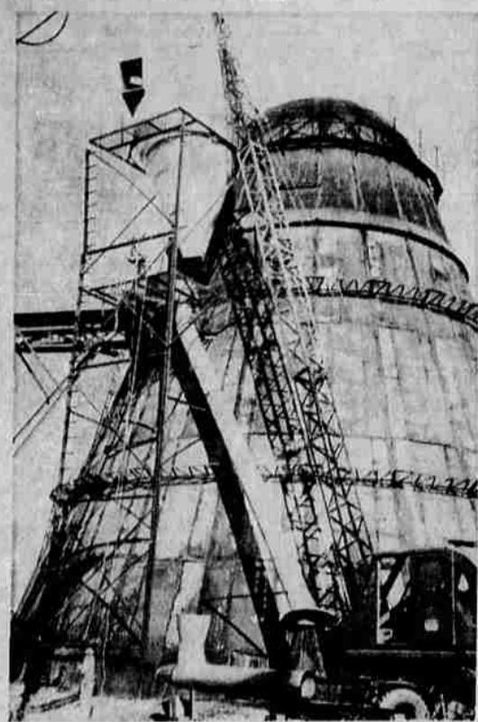
DISMANTLE CYCLONE —Al Avey, of Avey Brothers Lumber company, Kettle Falls, Wash., is shown cutting the cyclone from the sawdust burner at Moore Planing mill in Grants Pass. The cyclone is on its way to Kettle Falls, Wash.
