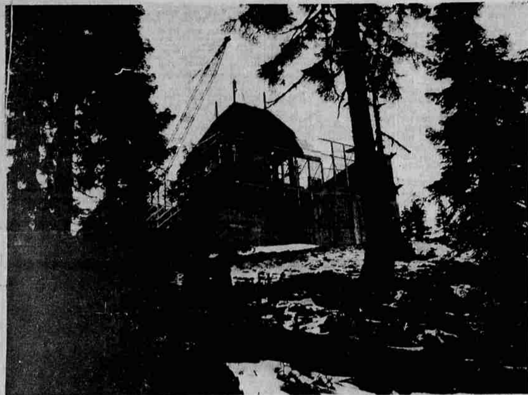
ONE UP, THREE TO GO—The first of the four towers that will adorn the top of the Mt. Ashland Ski Lodge was put in place by a large crane yesterday morning. The 30-ton crane, brought in from Eugene for the project, hoisted the 22-ton tower into place. Then workmen secured the tower onto the rest of the structure. This is how the scene appeared as the
