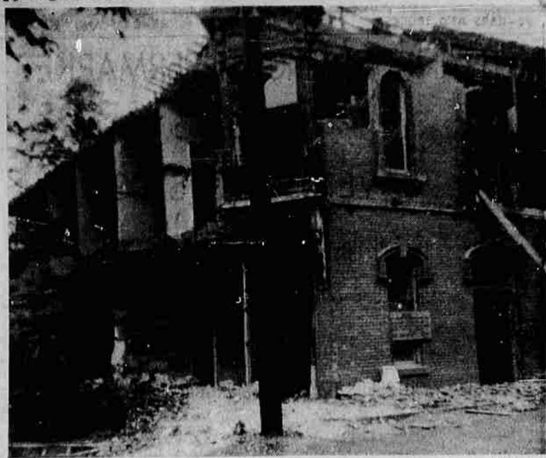
COMING DOWN—Don and Jean Fulcher of Medford purchased the old T. Jones Hotel in Hornbrook recently and started tearing it down and selling the old bricks of which the structure was built. This photo shows the demolition as it was in progress.
