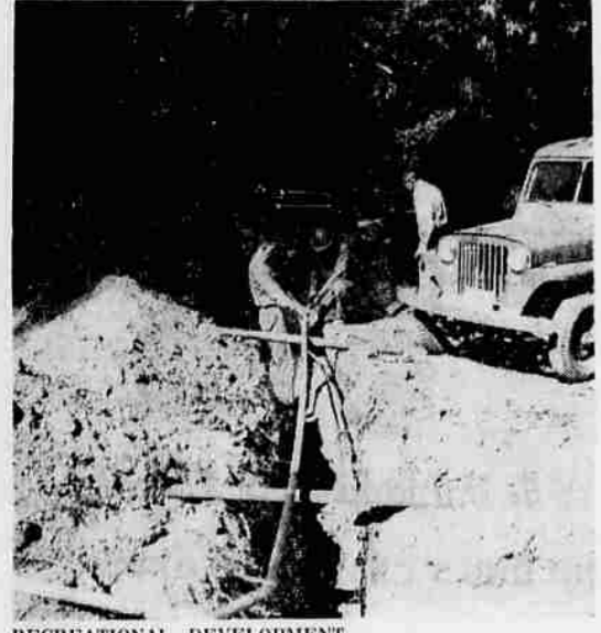
RECREATIONAL DEVELOPMENT Photo shows late summer installation of water system at Cook and Green Forest Service Guard Station on Middle Fork Tributary of the Applegate. The system was installed under supervision of Gene Cardwell, guard at Cook and Green, and was part of a rehabilitation program carried on there and at Beaver-Sulphur Camp. The program was planned when a forest recreation survey was made in '59 and '60. The survey was nationwide, and projected recreational needs of the public until the year 2000. New roads have been constructed in the camps, and next year additional camping units will be established.
