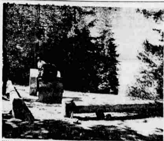
FINISH PAVING — Workman with a heavy roller is shown putting the finishing touches on campground paving project at Diamond Lake. The largest in the Pacific Northwest region of the Forest Service, Diamond Lake campground receives heavy summer use. (Forest Service Photo)
