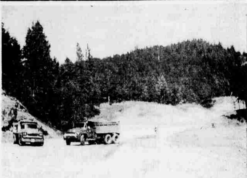
ROAD AROUND PROSPECT — The 6.5 mile bypass highway around Prospect continues to shape up, as workmen on the Federal Bureau of Public Roads project make gradual headway. This scene, taken in the Cascade Gorge area, depicts the wide roadbed that is being cut through a hilly area. At last report, the road was scheduled for completion sometime next year. It will run west of the present Highway 62, leaving the old road at Cascade Gorge and rejoining it just north of Prospect.
