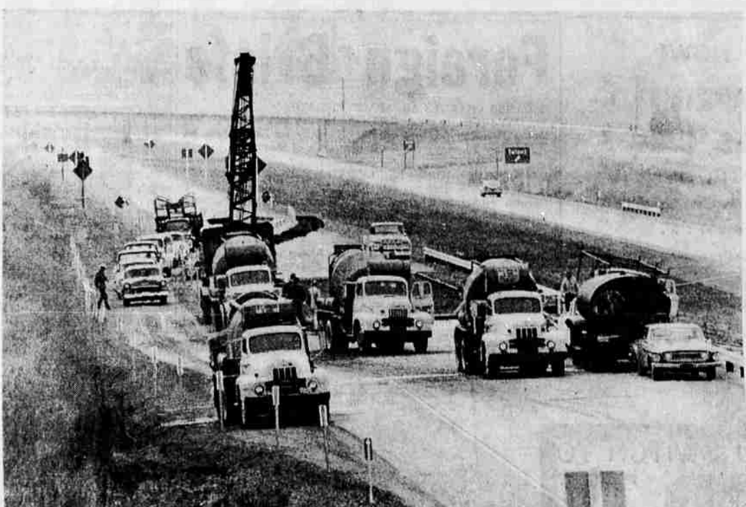
REPAIR FREEWAY—A section of Interstate 5 near the Talent exit, measuring about 150 feet, is being replaced and traffic is being detoured during the construction period. The section did not meet state specifications, Don Haller, resident engineer for the state highway department, said today, and it is being re-
