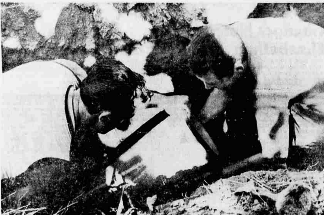
Each section of sewer pipe fits snugly into the next. To seal the connection, however, workmen put a rubber ring around the end of the section.
