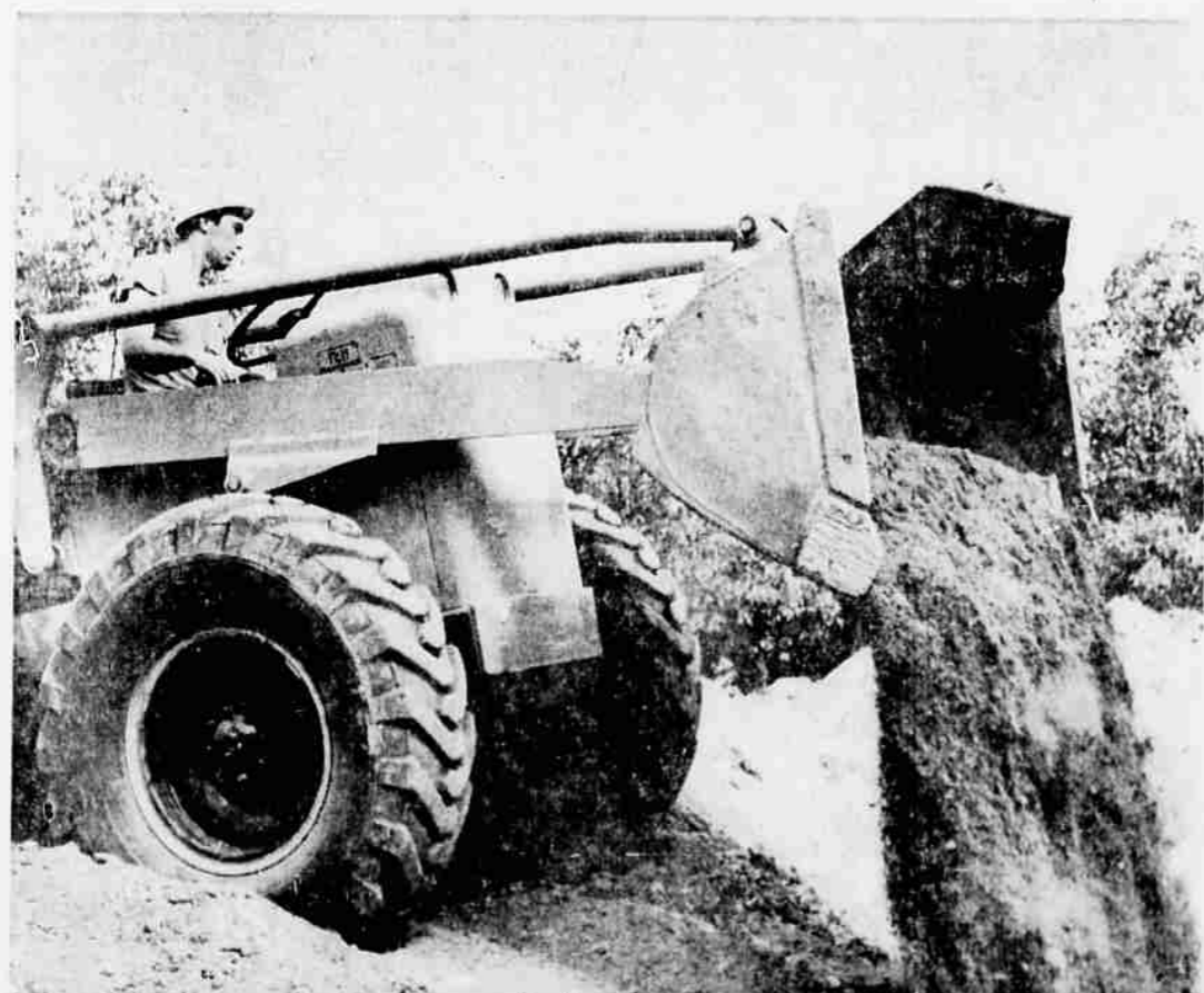
After the pipe has been laid and inspected, next comes the job of putting all the earth back into the trench. Workmen try to replace the earth as quickly as possible in order not to inconvenience residents any more than necessary.
