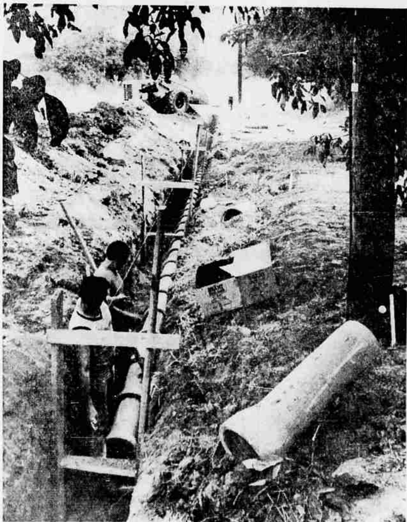
After the trench is dug, workmen lay the main sewer pipeline along the bottom of it. Here workers inspect a line being installed along California st.
