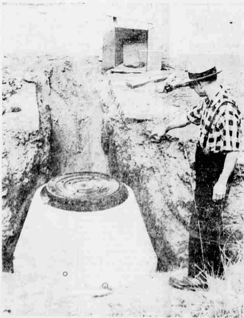
In order to avoid having to dig a new hole in the event of a malfunction in the pipeline, a manhole is constructed at every joint in the sewer system and also at various intervals along the lines. Councilman Paul Godward looks over one of them.
