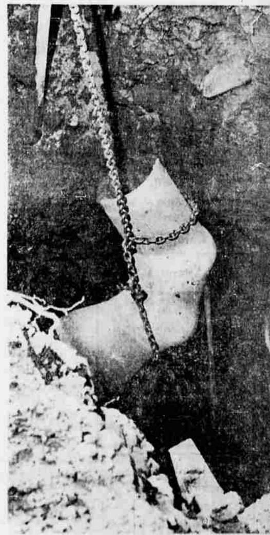
Construction workers here are lowering a section of pipe to be used at a joint in the system where two lines come together. Later a manhole will be constructed on top of the joint.
