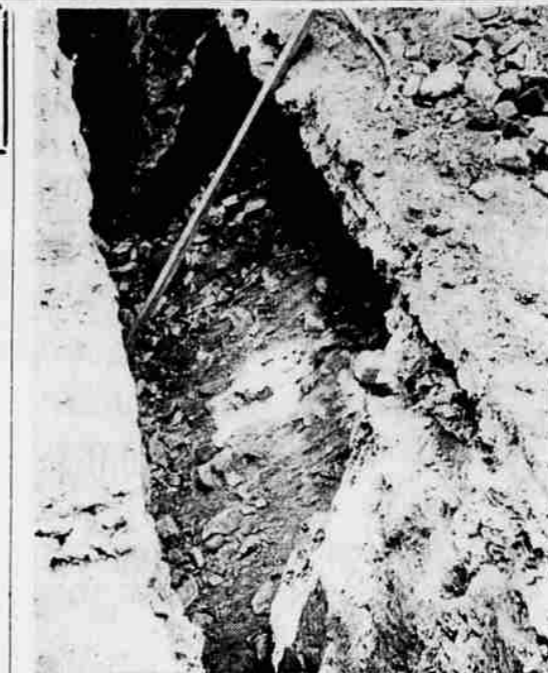
CISTERN UNCOVERED—One of the three old cisterns underneath Jacksonville was uncovered earlier this week when a sewer system trench being constructed across California st. at Fourth st. cut through part of it. The cistern may be seen just under the shelf at right. It originally was walled with brick and was used to store water for fire fighting.
