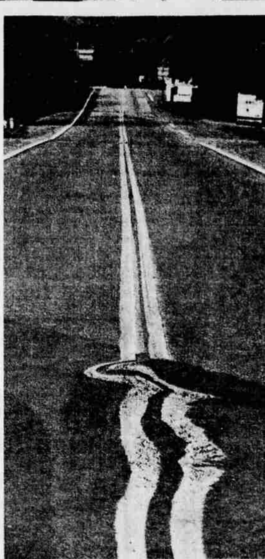
WHERE'S IT GOING? — Did he sneeze or did a blonde go by? This unusual highway center line makes one wonder as he drives over Route 12 near Bartonville, Pa. The unique design is on a repair patch on an overpass and might have been caused by a bump shaking the paint cart — maybe. (UPI)
