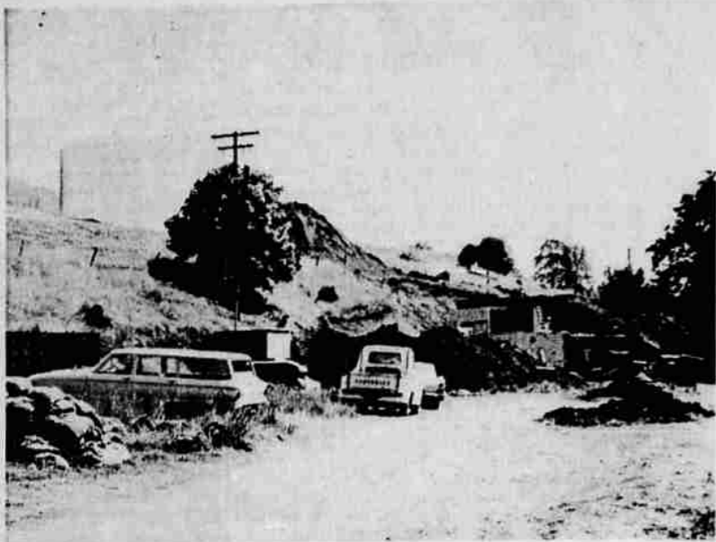
CONSTRUCTION PROGRESSES—Work on the new water system for the city of Talent is progressing rapidly. The water tank to be used for storage may be seen on the top of the hill at right in the above photo, while at left is the treatment plant under construction. When completed, the new system will give Talent a larger supply of water than is available at present. Water will be taken from Wagner Creek. The city's present source is a series of wells.
