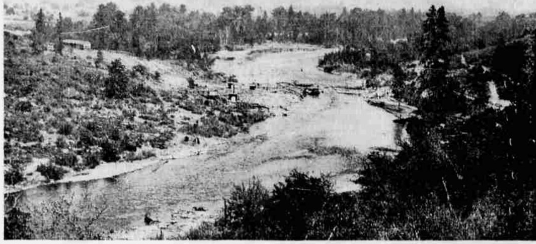
The coffer dam, constructed to open the way for installation of Gold Ray dam, was being built when this photograph was taken at the bend in Rogue river with the lower Table Rock in the background. On the right is the railroad crossing sign. The Southern Pacific line was given steady patronage by the Rays.
