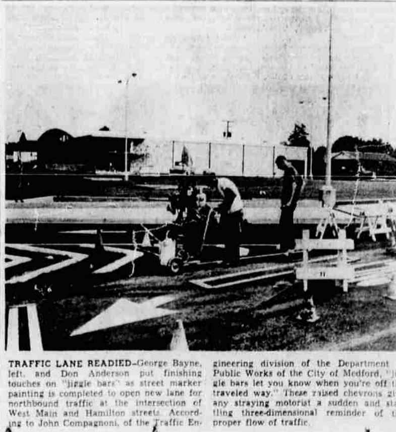
TRAFFIC LANE READIED - George Bayne, left, and Don Anderson put finishing touches on "jiggle bars" as street marker painting is completed to open new lane for northbound traffic at the intersection of West Main and Hamilton streets. According to John Compagnoni, of the Traffic Engineering division of the Department of Public Works of the City of Medford, "jiggle bars" let you know when you're off the traveled way. These raised chevrons give any straying motorist a sudden and startling three-dimensional reminder of the proper flow of traffic.
