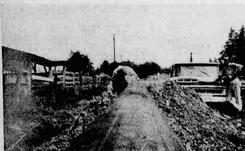
Welder, Harold Parris, puts the final weld on the two joint ends, which will be x-rayed by a technical process similar to "magnaflex" as used in oil fields.
