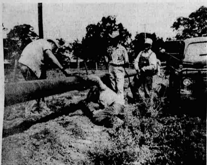
Tacking and aligning the joint, from left to right, Corbin Bland, pipe aligner; Pal Thompson, welder; Jack Derrick, Cal-Pac Utilities welding inspector; Charlie White, welder's helper.
