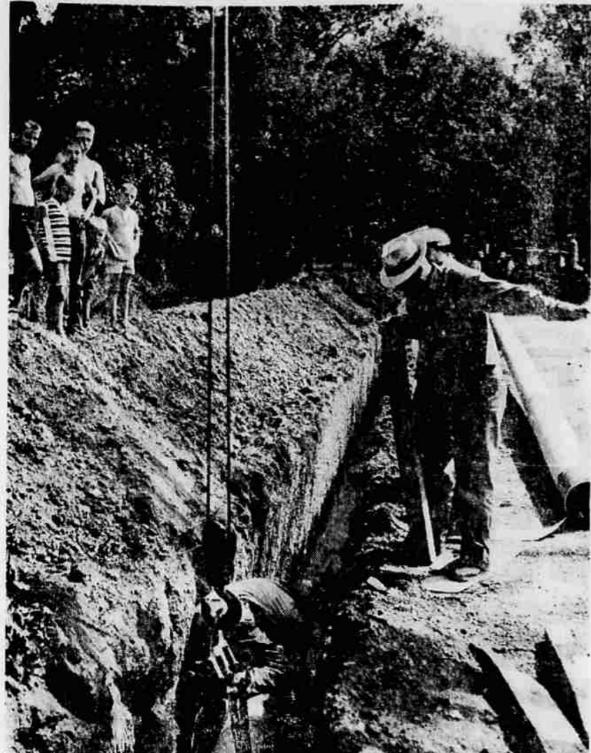
GAS PIPELINE - Work on the installation of the natural gas pipeline in the Rogue valley is progressing rapidly with crews installing the pipe on Perrydale ave. near Jacksonville highway Friday. California-Pacific Utilities company expects to have the pipeline in use by this winter. M. C. Lininger and Sons are contractors for the installing of two feeder lines in the Medford area. When the work reaches areas near homes workmen have an audience of neighborhood children.
