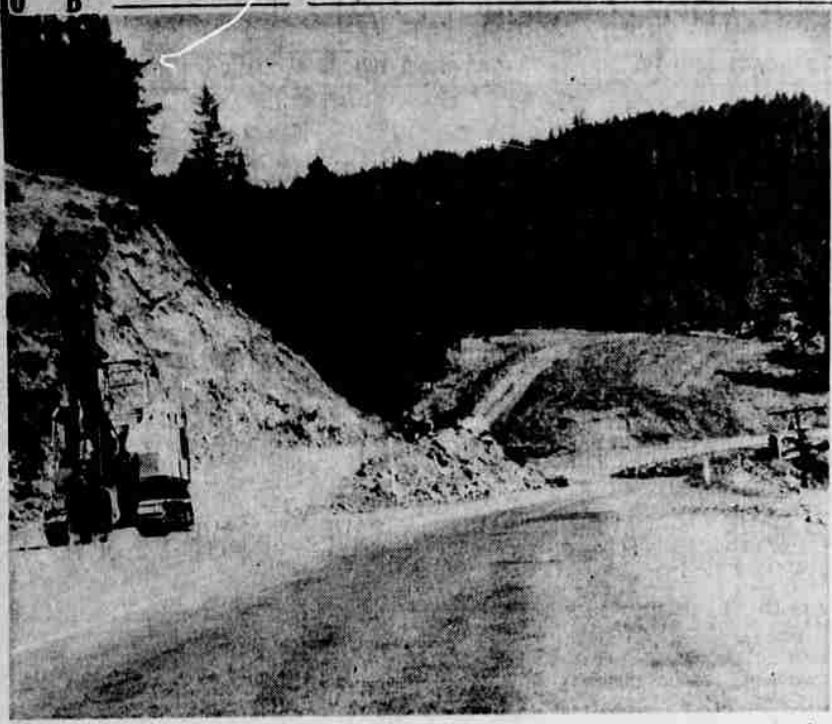
ROAD WORK NEAR PROSPECT - This picture shows where the new highway around Prospect will leave the present road at Cascade gorge. At right is the present Highway 82, while to the left of it is the road which has been cleared for the new 6.5 mile section which will bypass Prospect and the area south of it.
