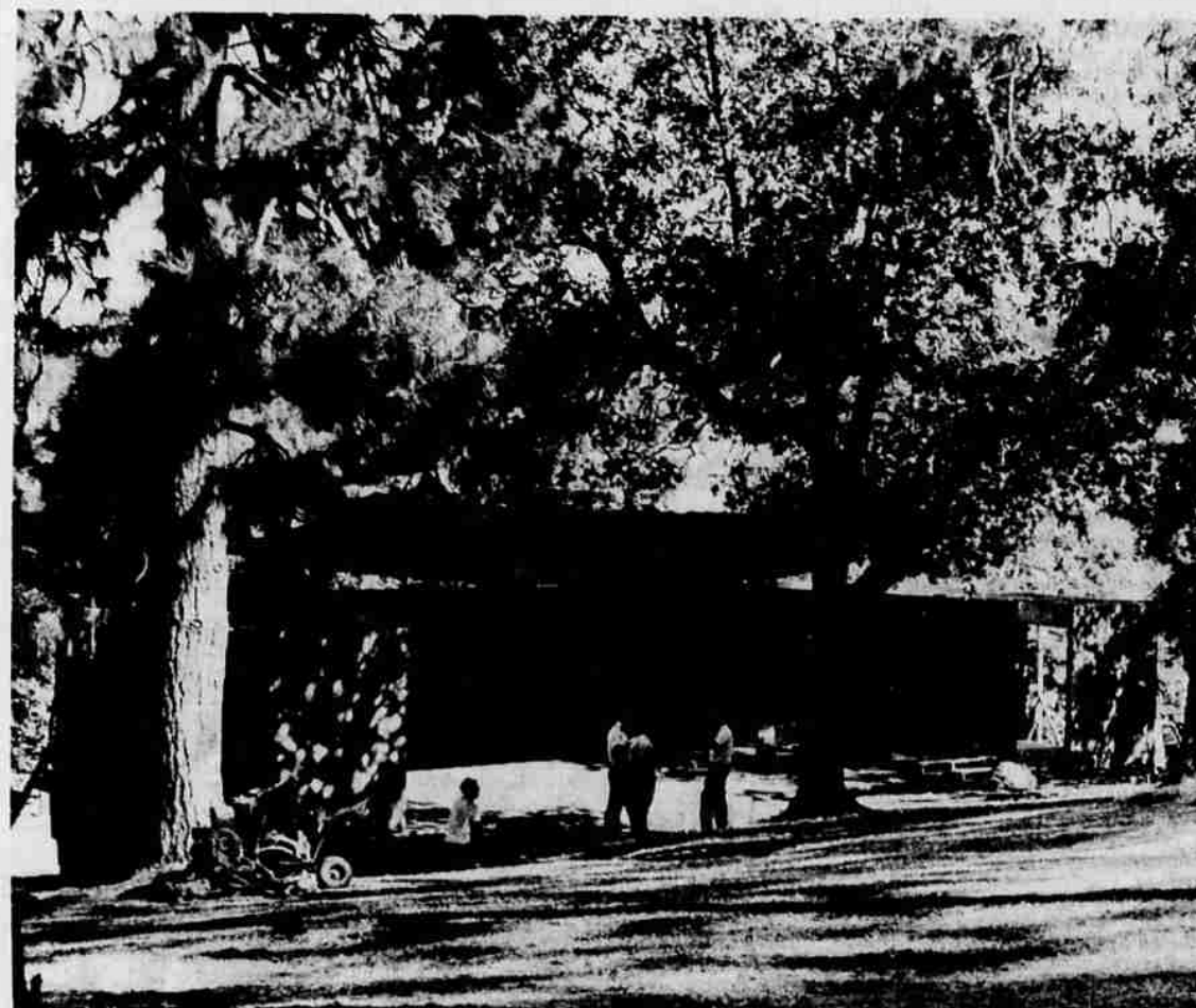
SHELL COMPLETED—Plans for the first annual Britt Music festival in Jacksonville are nearing completion. Construction of the shell is completed and ready for the musicians. The first concert will be given at 4 p.m. Sunday. A benefit champagne reception to honor the orchestra members will be held from 7 to 9 p.m. Saturday at the shell. The public has been invited to attend the reception.
