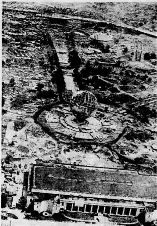
WORK PROGRESSES —The Unisphere, center foreground, global symbol of next year's New York World's Fair, seems to have all of its continents now as work progresses at the Flushing Meadows site. (UPI)
