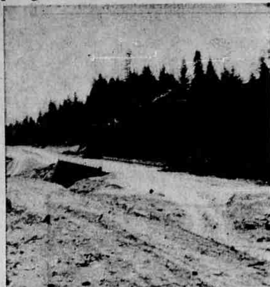
HIGHWAY SHAPING UP—A sign of the progress being made on the new road around Prospect is this bridge over the Rogue river which recently was constructed. The road involves about 6.5 miles, leaving present Highway 62 at Cascade gorge and rejoining it north of Prospect. The road will run to the west of the present highway.
