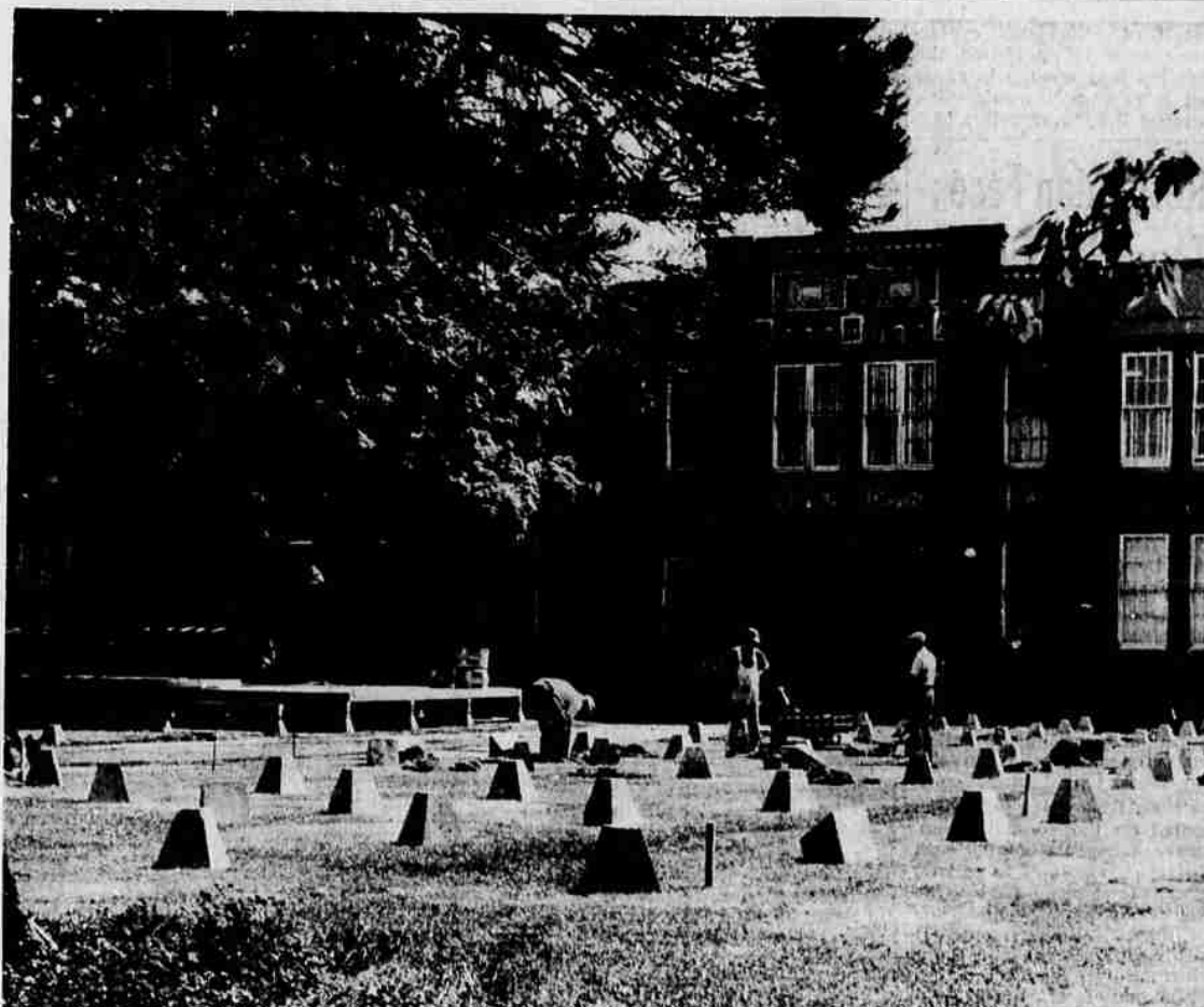
BUILDING STARTS —Installation of six temporary classrooms at Medford High school started recently. Here district workmen are preparing concrete blocks which will hold the buildings. They are scheduled to be ready early next month when school starts.
