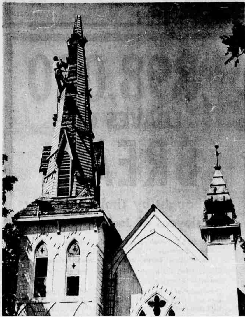
STEEPLEJACK AT WORK —A church in Jacksonville is catching the eye of tourists these days. High up on the First Presbyterian church's steeple, approximately 80 to 85 feet high, works a steeplejack. The contractor, Milton Wallace, is replacing the original wood shingles that were put in
