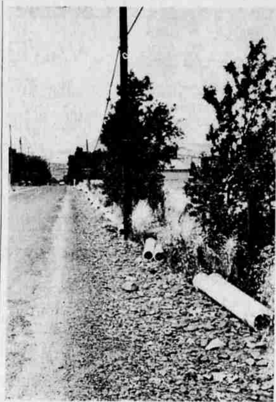
PIPELINE FOR THE NEW SYSTEM —Lengths of pipe are shown along Wagner Creek rd. near the Talent city limits as workmen last week were laying the main pipeline which will bring the city's water in from the treatment plant to users. Starting from the plant site, workmen have been digging a ditch and laying the pipe, gradually working toward the city. The ditch had not yet been extended to the part of Wagner Creek rd. shown above when this photo was taken.
