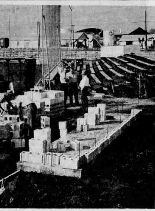
DUGOUTS - Construction of the new dugouts for Jackson County fairgrounds is being carried out by local Bricklayer's Union No. 9 and other local groups. Materials used in the buildings were donated by local business firms.
