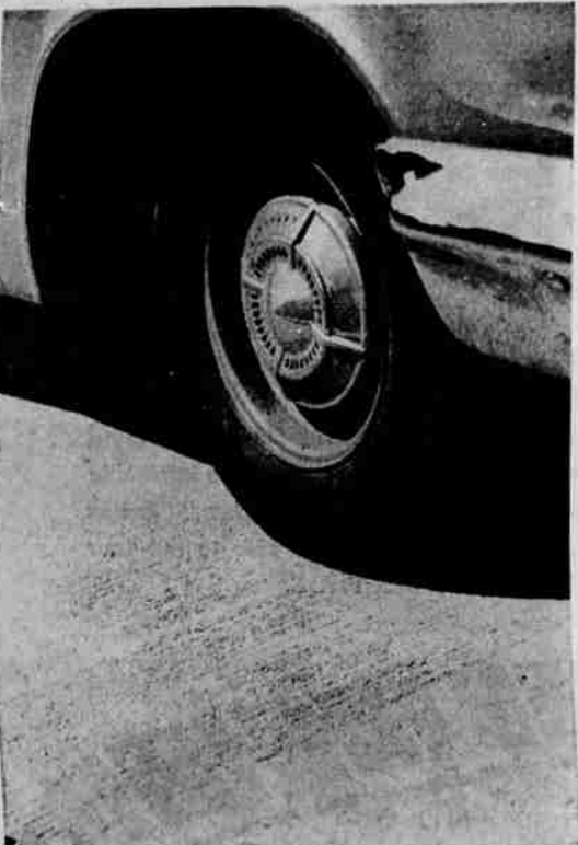
SHOWS SURFACE—This picture illustrates the surface of the new section of Interstate 5 between Medford and Ashland. It is designed to be a non-skid surface along the continuous section of concrete pavement. (Knackstedt Photo)
