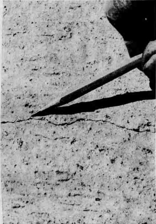
SHOWS CRACKS—This picture shows the size of the cracks on the continuous stretch of concrete on Interstate 5 between Medford and Ashland. The hairline cracks eliminate joints every 66 feet along the highway. (Knackstedt Photo)
