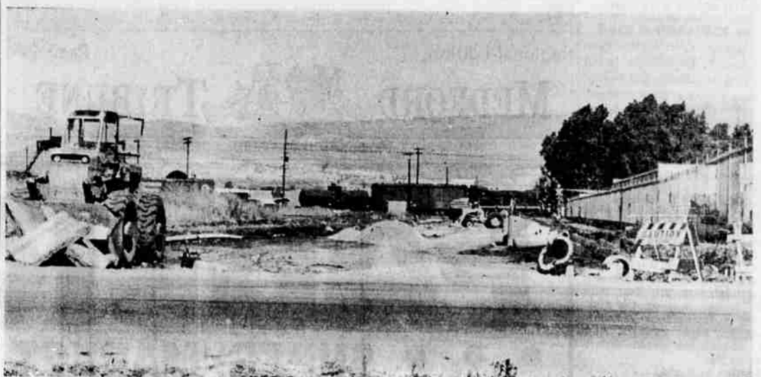
BARNETT ROAD EXTENSION —This photograph, taken from the west side of Grape st. looking east, shows equipment of M. C. Lininger and Sons at work on the extension of Barnett rd. The firm was awarded the $2,757,253 contract for the project by the Medford city council. Completion date is scheduled for Sept. 30, according to Vernon
