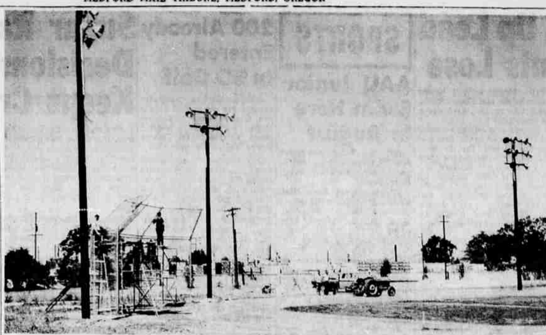
NEW BALL FIELD — This is the new lighted ball field at Jackson park. It is scheduled to go into use Wednesday, July 17, with two games of the Jackson County Softball association. Here the backstop is being completed and work is being done on the new dirt in the baseline area. — (Knackstedt photo).
