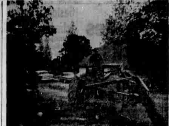
IMPROVE WATER SERVICE - Workmen were on the job last week digging ditches to accommodate completion of the "loop" of water line connecting Seventh st. with North Broadway in the city of Rogue River. The line being installed is a four-inch transite pipe. When complete, city officials reported, it will give better water service to the residents of the North Broadway and Valley View dr. areas.
