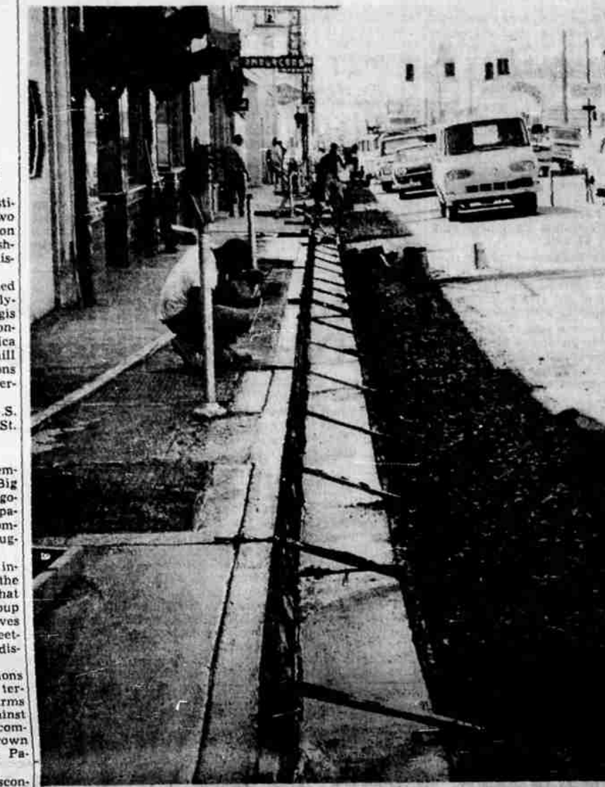
INSTALL NEW CURBS—Contractor's crews are shown here this week installing new curbs and gutters at Main st. and Riverside ave. The work is part of a project jointly financed by the city of Medford and the state highway department...
