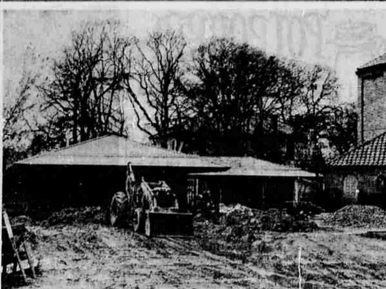
NEARING COMPLETION—The new rectory at Sacred Heart Catholic church on South Oakdale ave. is nearing completion. The structure will provide a study, bedroom and bath for each of the four priests plus a guest room. The present rectory, the two story white building on the property to the south of the church, will continue to be used for housekeeper's quarters, dining room, kitchen, and office space. A second unit on the new structure, to be built at a later time, will provide for these facilities and the old building will be torn down.
