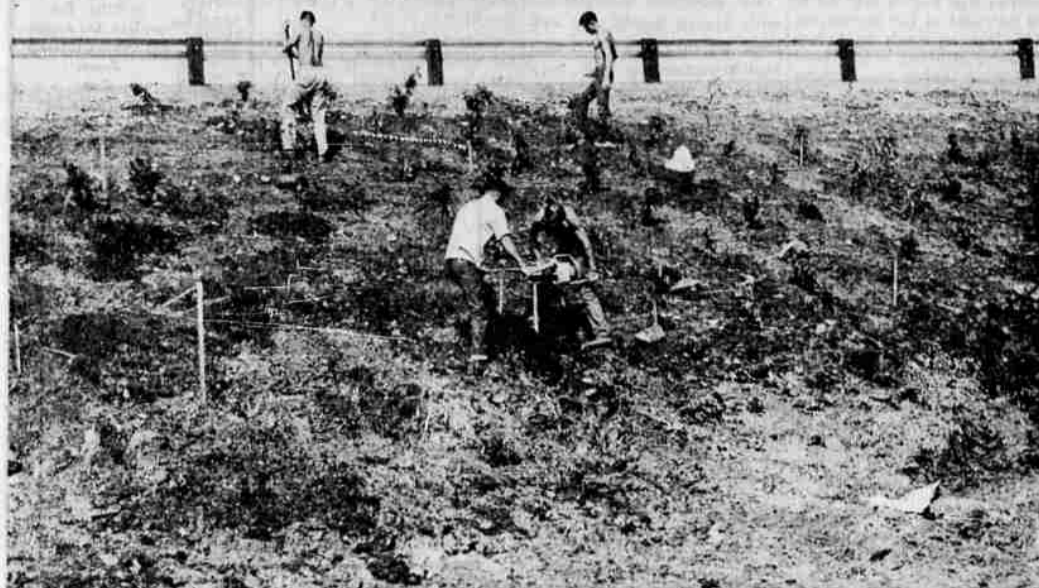
INTERCHANGE BEAUTIFICATION—Crews are busy planting shrubs and trees at the Crater Lake highway interchange of Interstate 5. Landscaping at the interchange is under contract to the Aichele Landscaping firm of Portland. Among shrubs being planted are Chinese and macrantha azaleas, tamarix and anadonna creeping juniper, glossy abelia; H. E. Beall, King George spring and golden fitzer heather; Katherine Dyke's, common bluebeard and war-minister broom. Trees include silk, ponderosa pine, honey locust, scarlet oak, morine honey locust, and Portuguese laurel cherry. Part of the area will also be in lawn, according to state highway department officials. The entire planted areas have underground sprinkler systems, which have already been installed. (Knackstedt photo)
