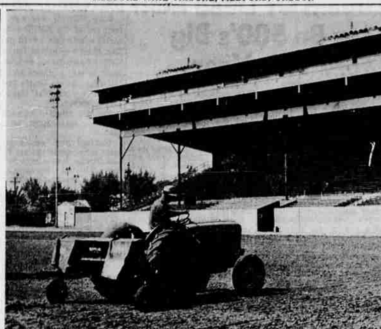
SEEDING THE FIELD —Seeding of grass on the Medford High stadium field, accomplished by workmen and equipment as pictured above late last week, has been completed. The workmen spread ground up bark mulch on the ground yesterday and this morning, and watering of the whole field was scheduled to begin tonight. The field is expected to be in shape in time for the first football game this fall. It will not be used for any summer activities.
