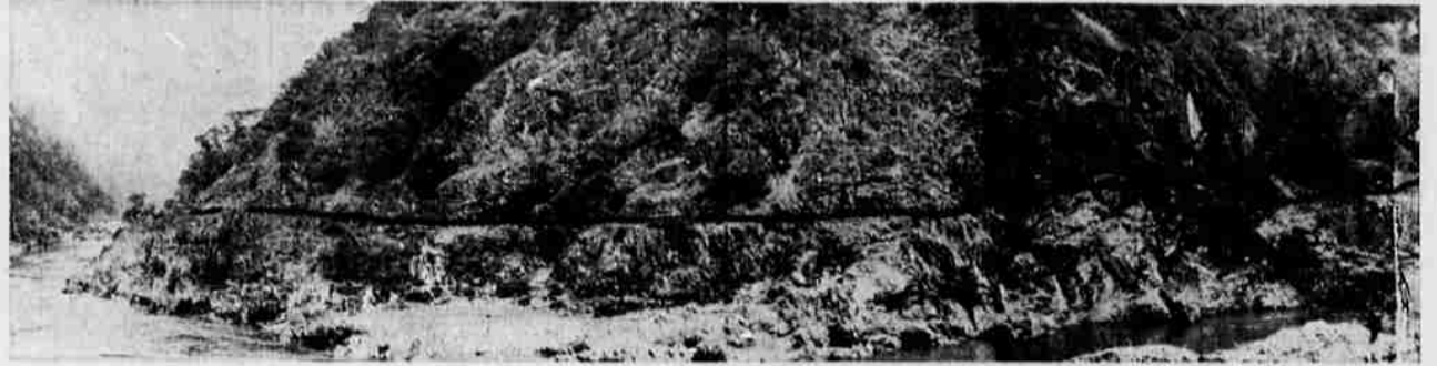
The black line on the edge of the cliff along Rogue river between Grave and Whiskey creeks shows the location of the new Rogue river trail, being constructed by the bureau of land management under the accelerated public works program in Josephine county. The new trail starts at the right of the top picture at a boat ramp near Alameda bridge, which is behind the trees to the extreme right of the picture. The new trail connects with an old trail at the extreme left of the lower composite picture by the bureau of land management. The pier of an old bridge across the river is located where the new trail connects with the old one at the left of the bottom picture. Pictures on this page, other than BLM composite picture above, were taken along the new trail last week.
