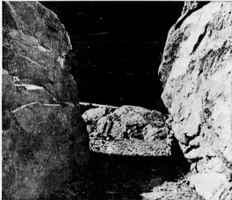
The new Rogue river trail, in some places, has been blasted out of solid rock, as at the location pictured above. When completed, the trail will provide access into an area where access has been limited.
