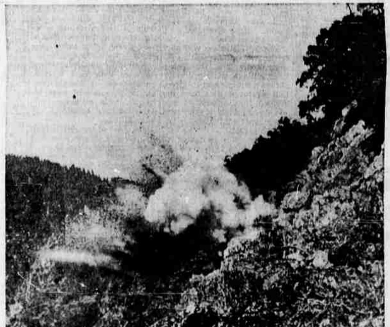
Explosives clear the way for much of the new four-mile section of the Rogue river trail on the north side of the river.
