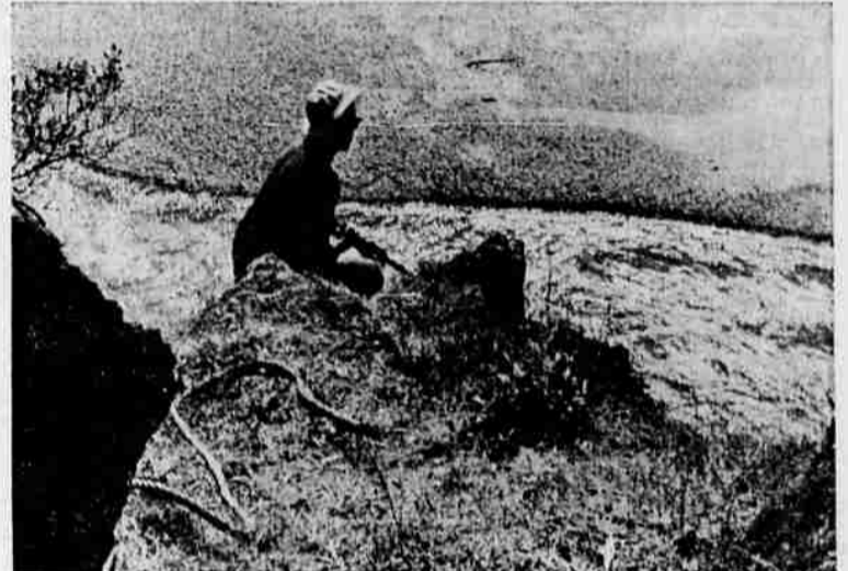
Phil Squires crouches on top of a cliff overlooking Rogue river breaking off rock loosened by a dynamite blast a few minutes earlier. The trail at this location will be about half way done.
