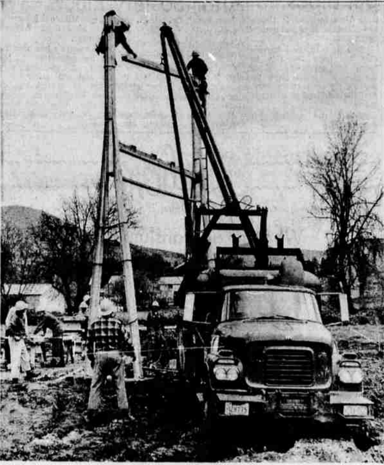
CONSTRUCT SUBSTATION —With aid of a big truck-mounted boom a section of the steel substation structure slides into place at Pacific Power and Light company's new Gold Hill substation. When complete, the $65,000 installation will provide for an in-
