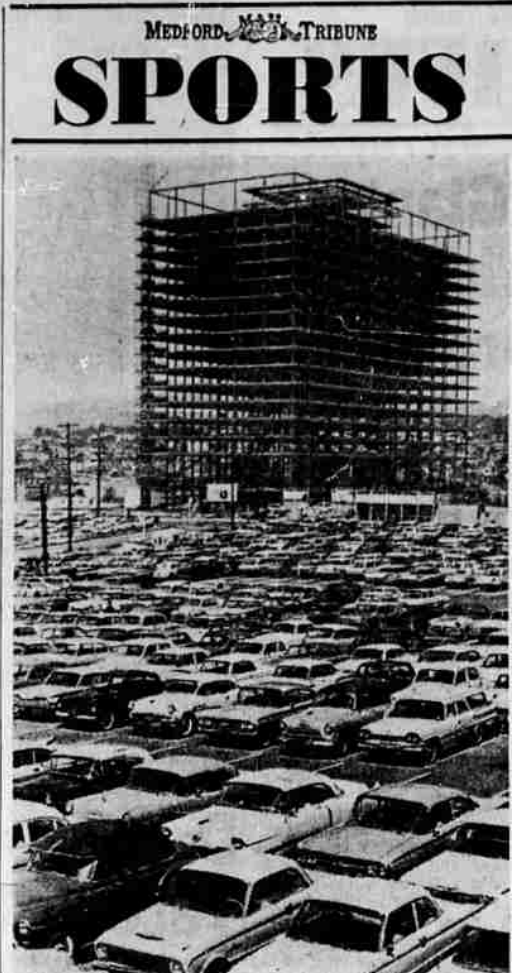
JAMMED WITH AUTOS—In Los Angeles, this new building goes up in back of parking lot jammed with cars of workers who drive to their jobs in the Civic Center. Los Angeles is one of the traffic congested cities cited by the Senate Banking committee in recommending passage of President Kennedy's bill for helping city mass transport systems. (UPI)
